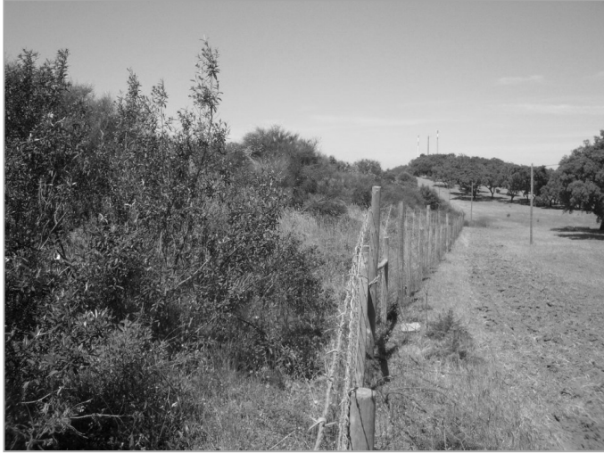
Fig. 6.2 – Example of a fence installed in the highway A6 verge to avoid livestock and wild boar ( Sus scrofa ) to enter the road area. Fence height is ca. 1.5 m.
