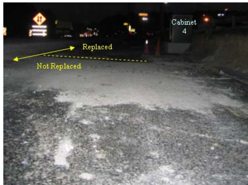
Figure 3.15 Region PCC slabs were removed and a portion of the ATPB was replaced.
