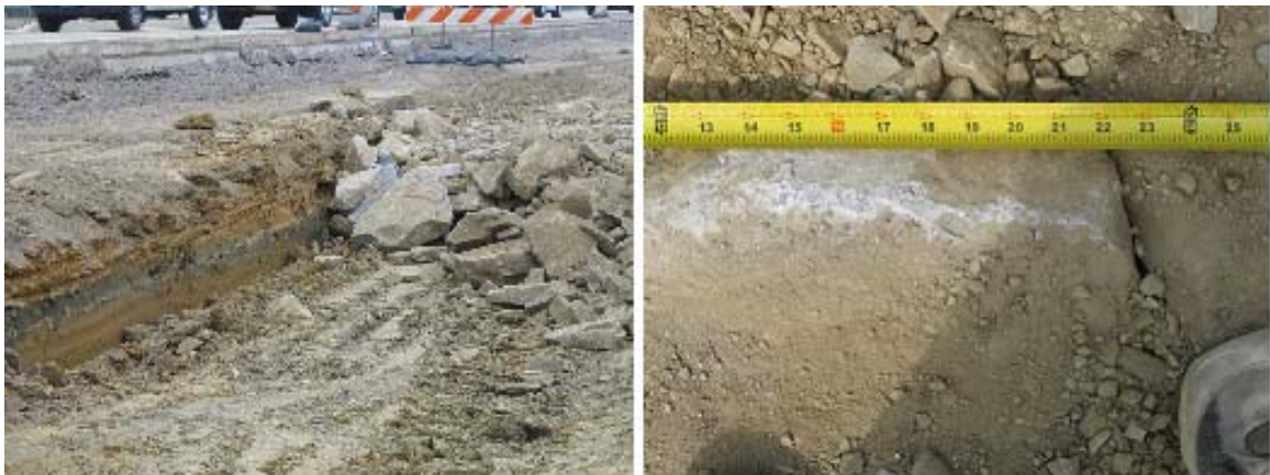
Figure 3.10 Backfill material containing large boulders.
