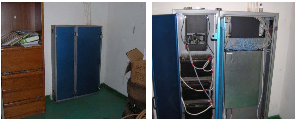
Figure 14: Steel cabinets housing server and battery system
