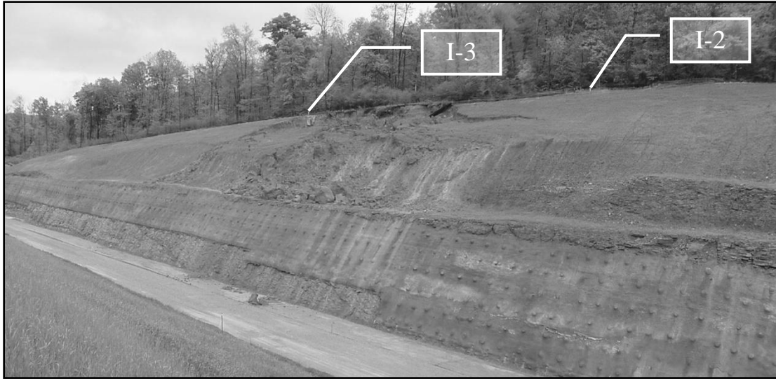
Figure 1.7. Clay Slope Failure.
