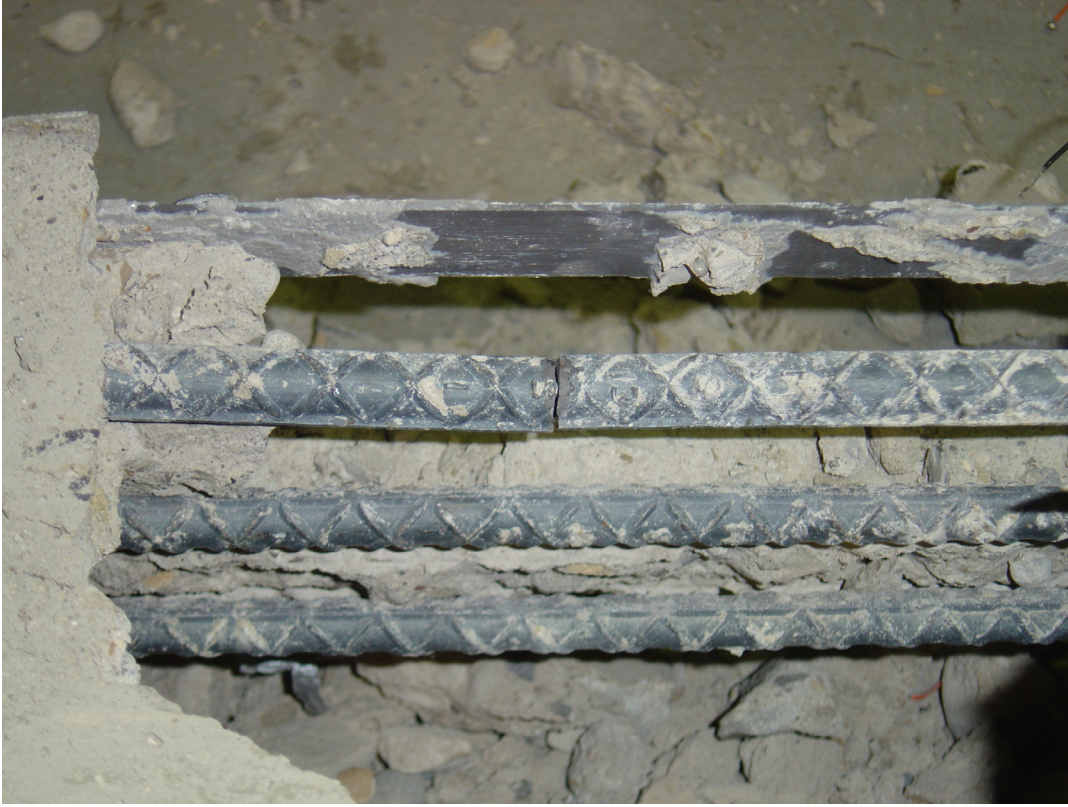
Figure 3-22 Typical fatigue-induced reinforcing bar rupture
