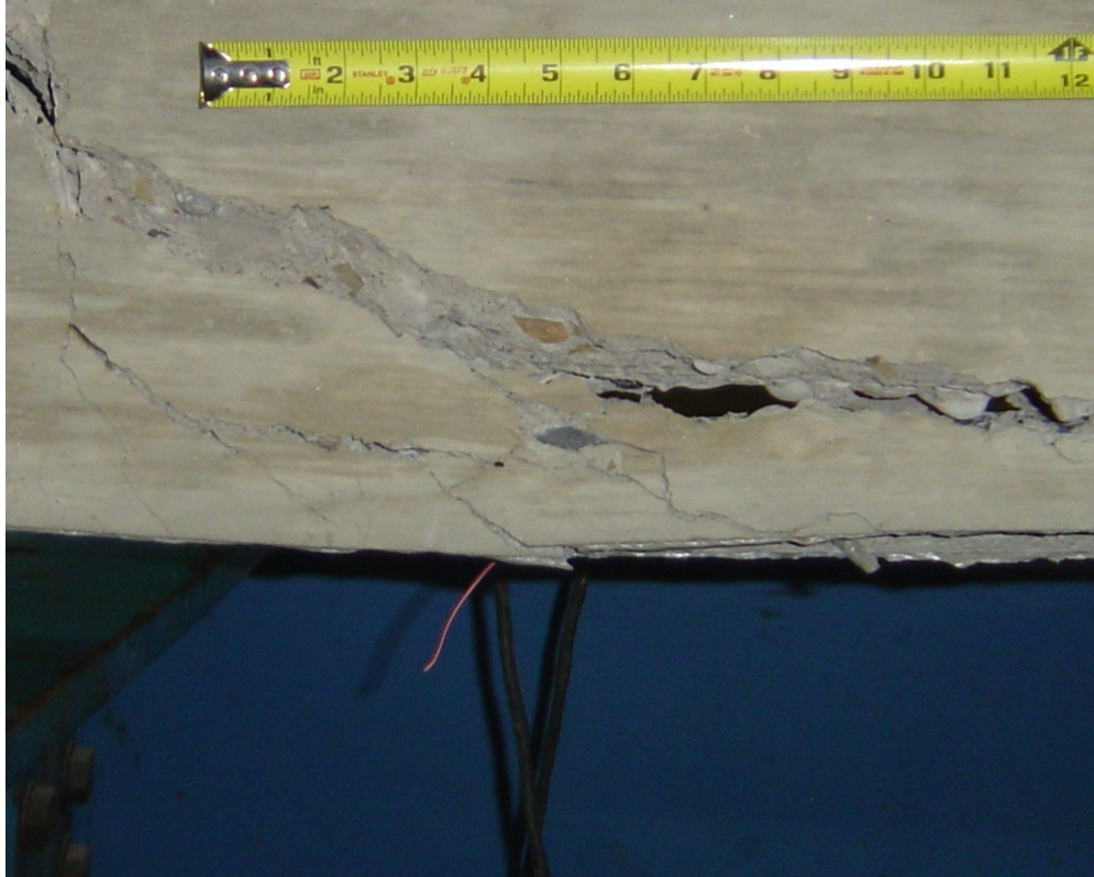
Figure 3-23 Representative debonding at toe of shear crack. (Splitting failure is secondary.)
