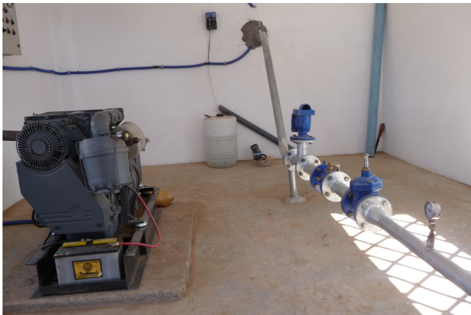
(B3) SAEP Motor Pump in a Cement Building in the Oasis of 'Àfra
