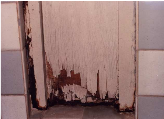
Figure 5.0: Rotting door due to moisture penetration effect door frames and panels
