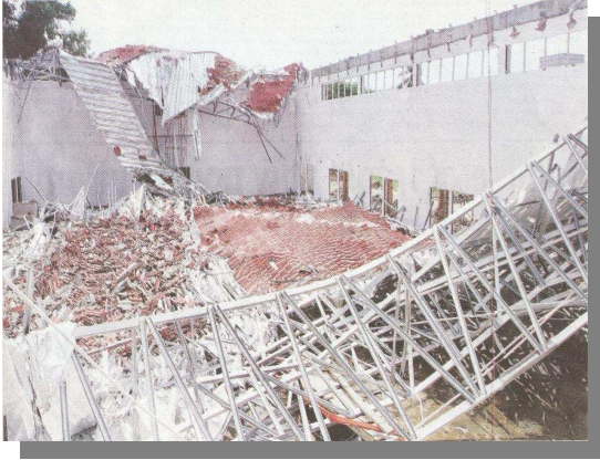
Figure 3.0 Roof structure collapsed in Kuantan (NST 2005)
