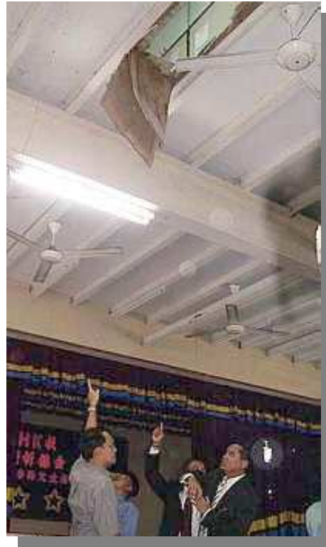
Figure 2.0: Second floor-board falling down due to termite problem in Ipoh. (NST, 2005)
