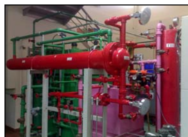
Figure 1 – The boiler drum and heat exchanger QAD Model BDT 921 (Real system)
