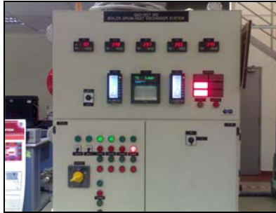
Figure 2 - The front panel control of boiler drum and heat exchanger QAD Model BDT 921 (Real system)
