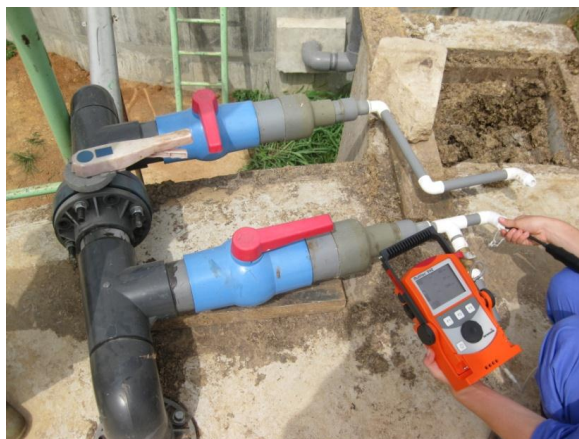
Figure 4.2. Biogas analysis of the gas from Digester 1 with a Sewerin Multitec 540 gas analyser.
