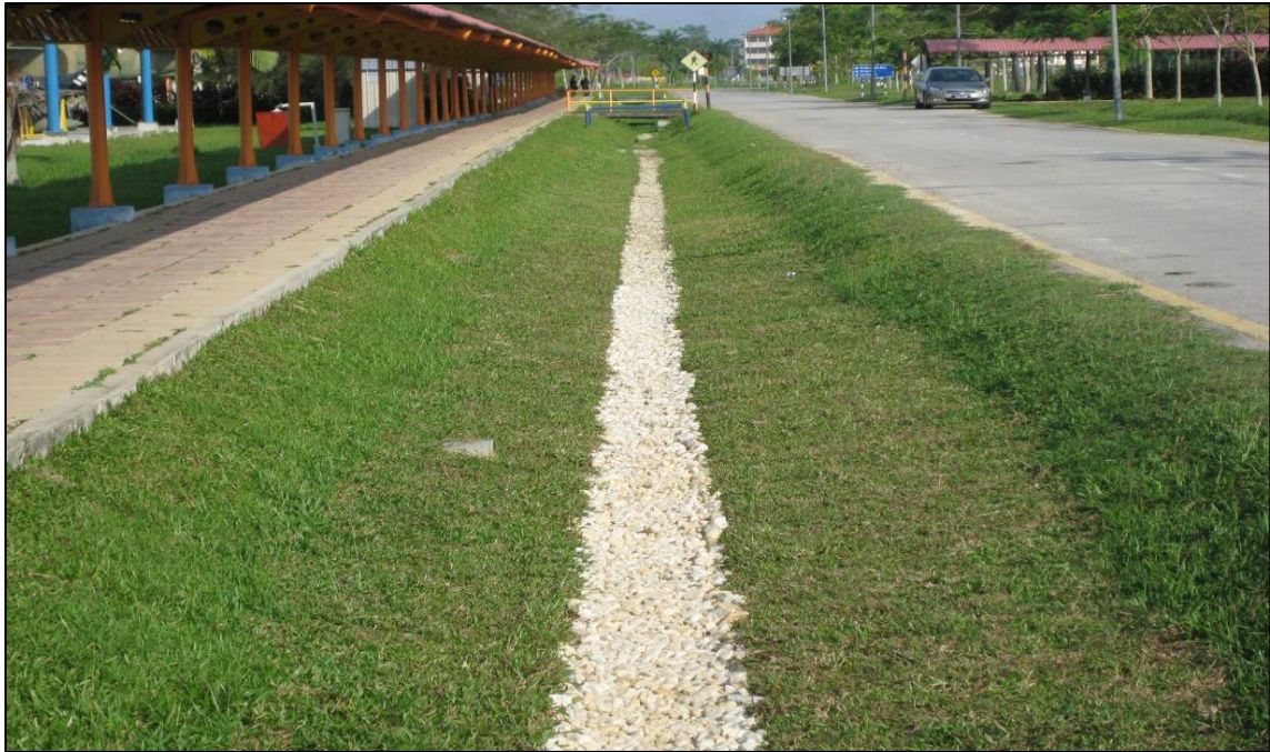
Figure 2. An ecological swale with river gravels making up the low flow channel.
