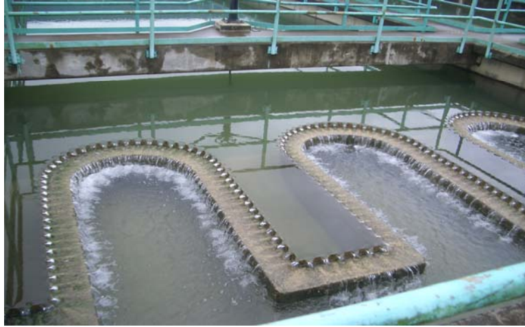
Plate 2.3: 'Finger' weirs collecting clarified water in sedimentation tank (With permission from the Segama WTP)
