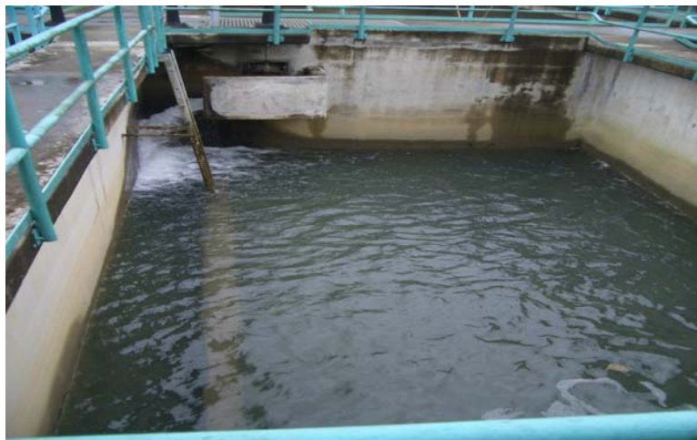
Plate 2.4: Rapid gravity filtration tank (With permission from the Segama WTP)
