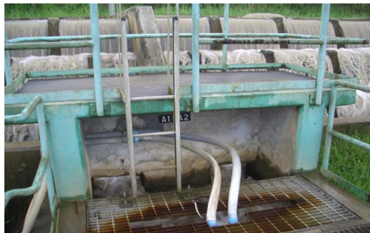
Plate 2.1: Aeration process and chemical addition (With permission from the Segama WTP)
