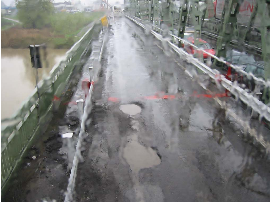
Figure 2 Pavement quality discontinuity The bridge over river Tisza between Záhony and Csop
