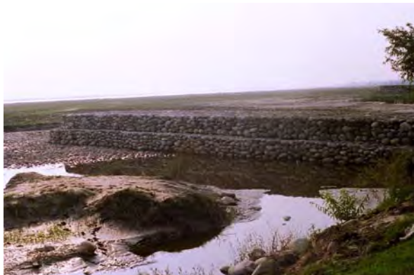
Embankments have been put up to control the water during heavy flooding.
