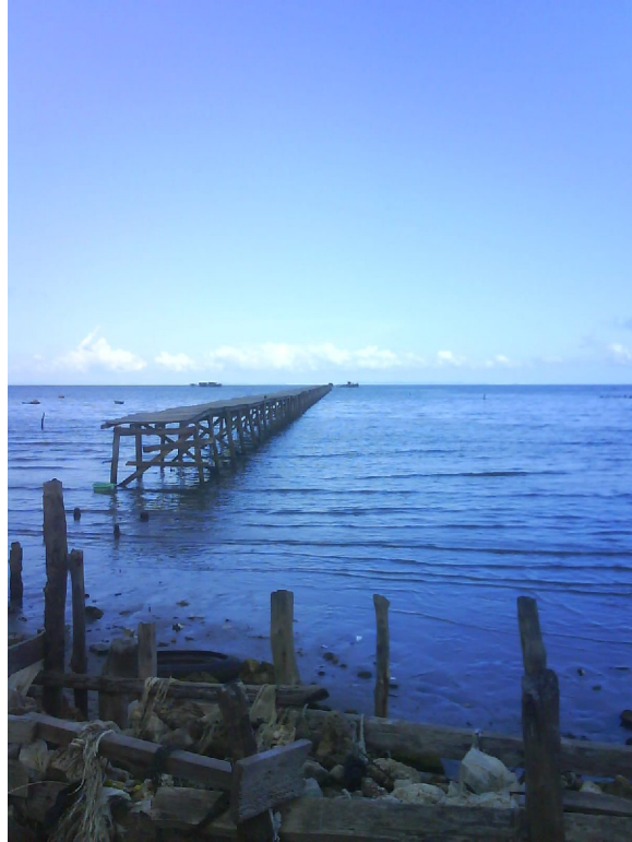
Figure 2.3: The delapidated state of infrastructure in Pulau Banggi.
