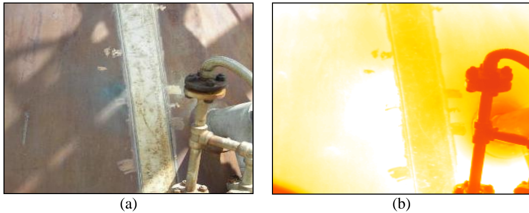
Figure 1.6 (a) Defective refractory incinerator and (b) its thermogram
