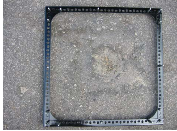
Figure 3b: Right image of delamination
