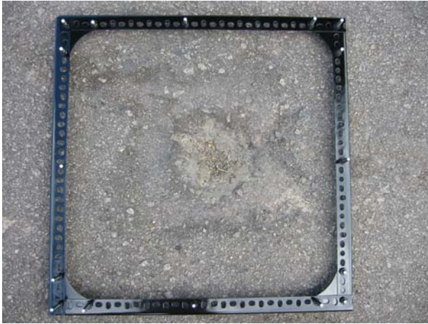
Figure 3a: Left image of delamination
