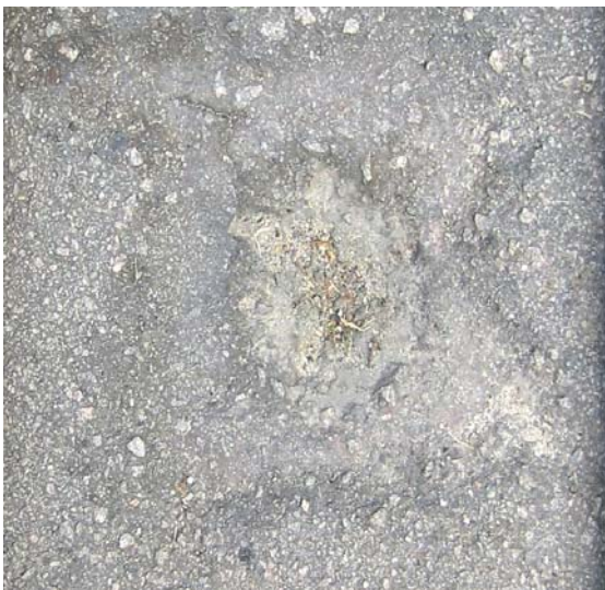
Figure 5: Ortho-image of delamination.
