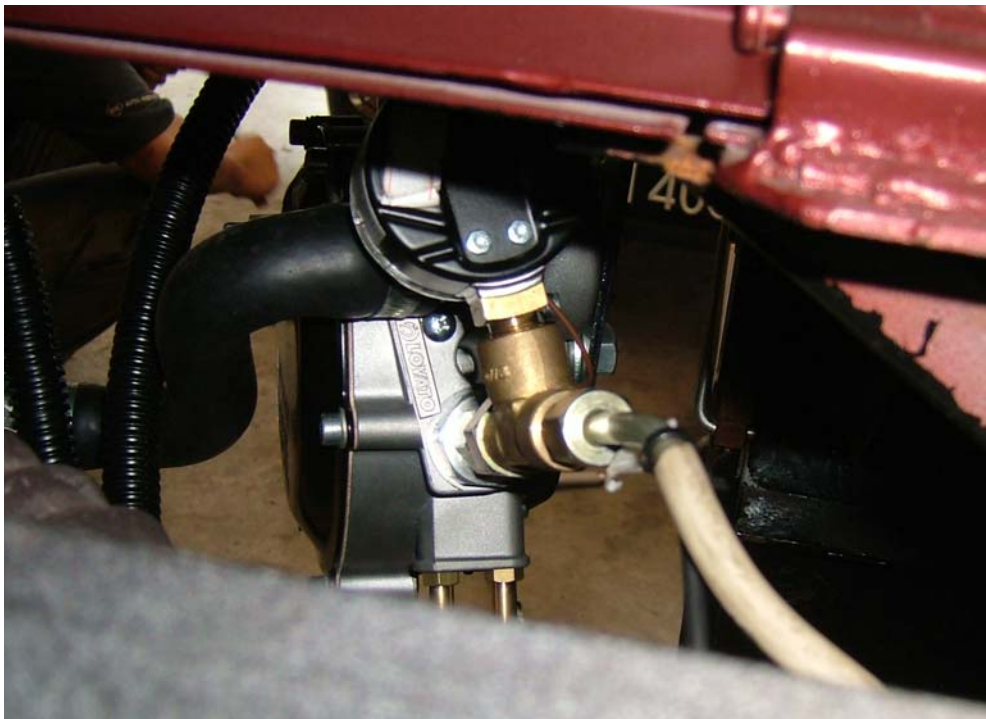
Figure 5.19: The pressure gauge connect to the high pressure pipe to monitor the pressure in the CNG tank
