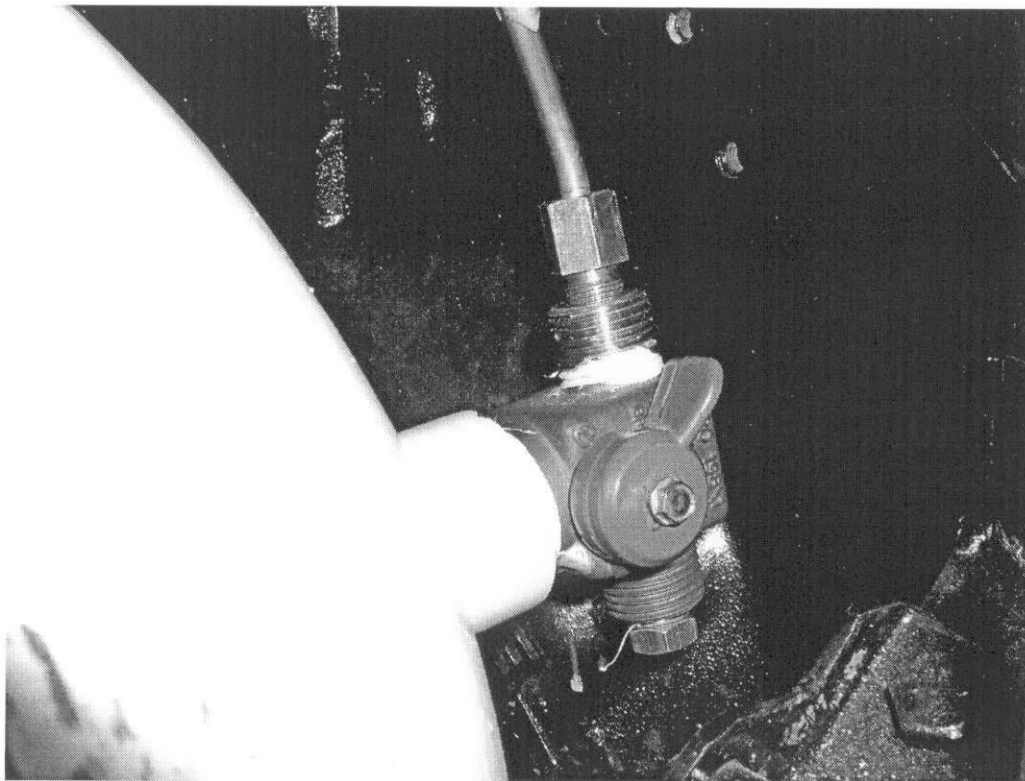
Figure 6.13: The emergency manual shut-off valve at the cylinder head
