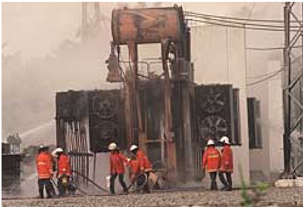
Figure 1.2: Example of a transformer explosion at a TNB sub station - 2
