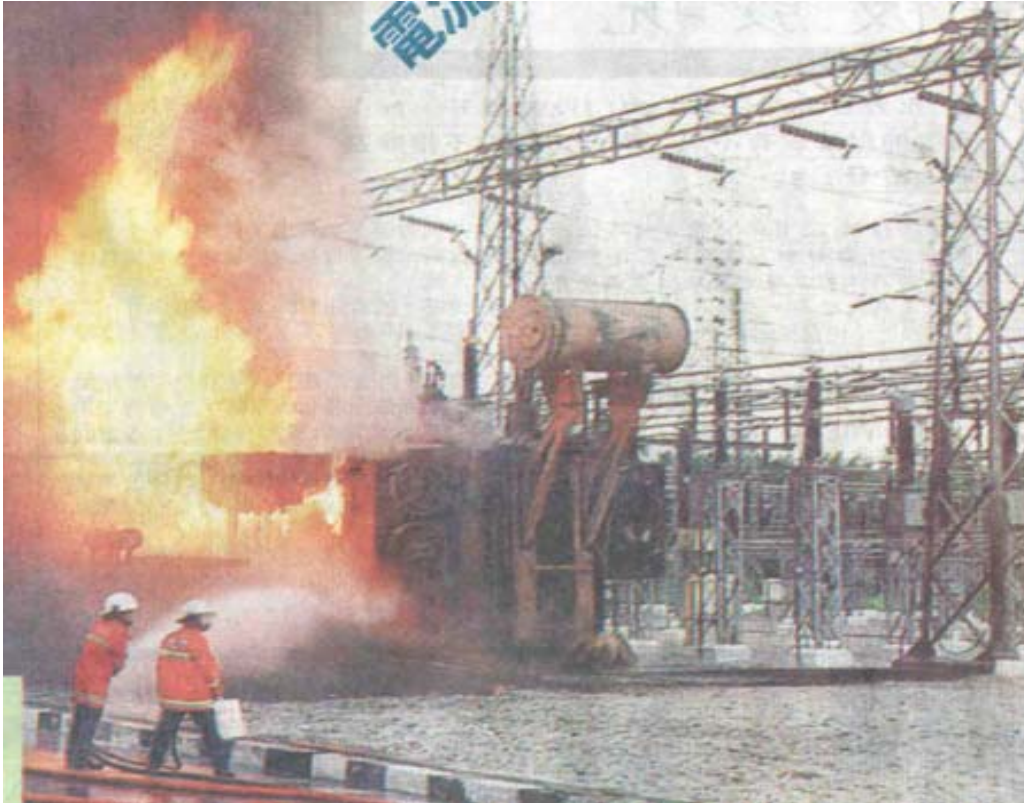
Figure 1.1: Example of a transformer explosion at a TNB sub station - 1
