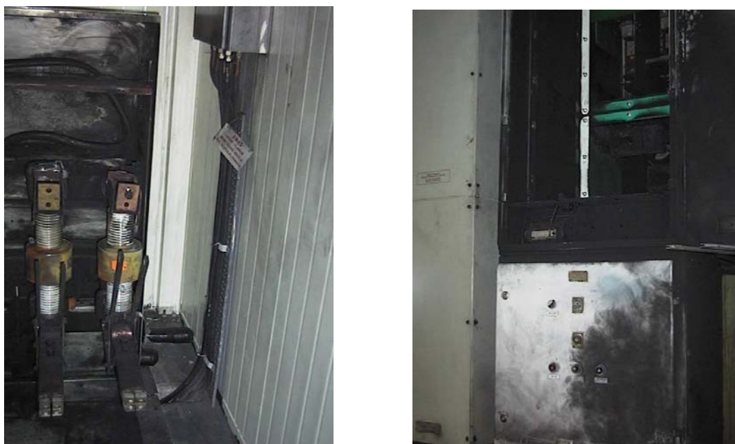
Figure 1.3: Consequence of transformer failure
