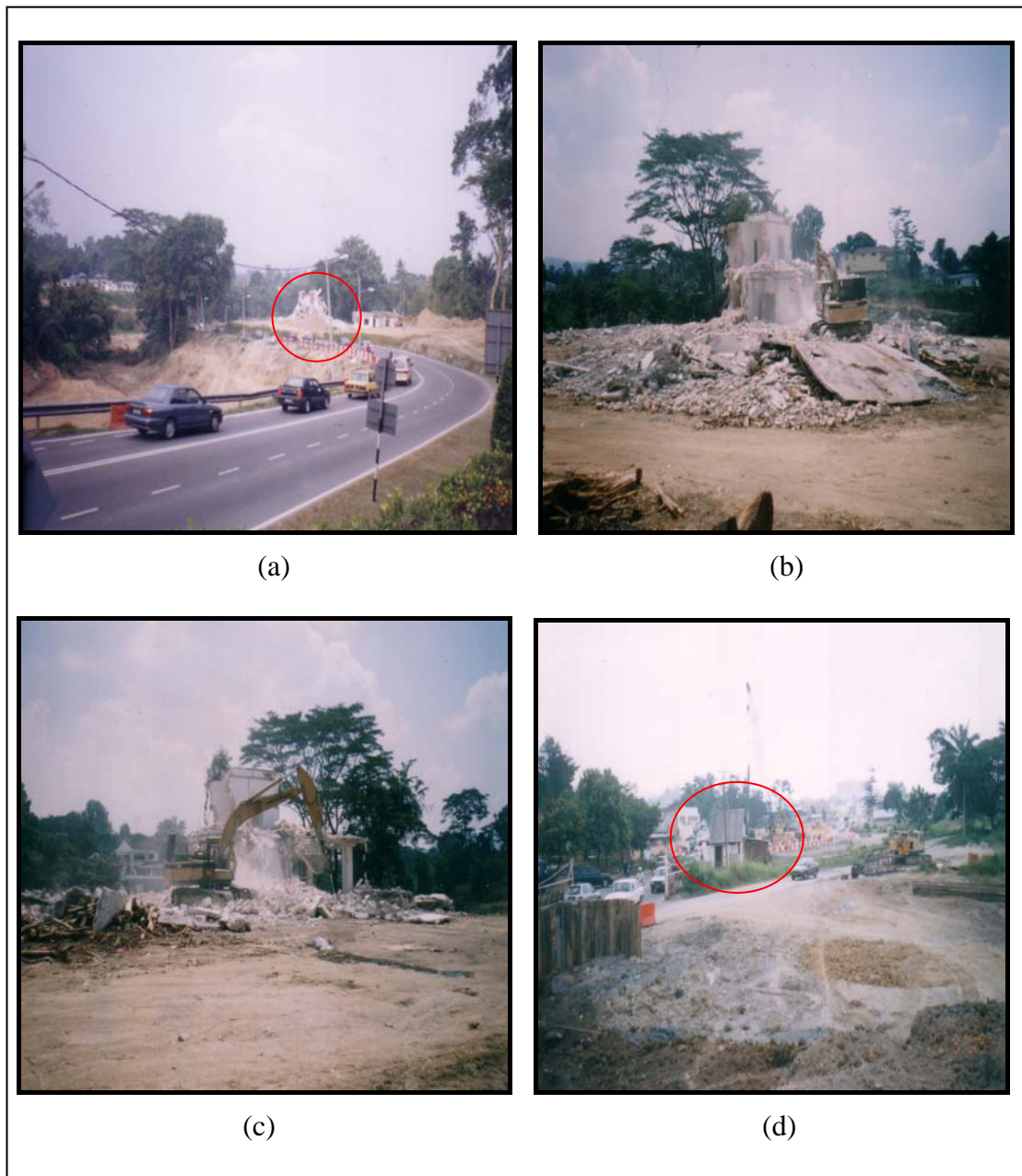
Figure D1 (a-c): Demolition works being carried out on a bungalow as part of the Jalan Lingkaran Tengah Project in Seremban, Negeri Sembilan; (d) All that is left standing after site clearance.
