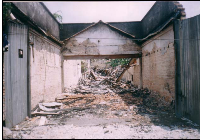
Figure D3: Structures damaged or destroyed by fire are frequently demolished to eliminate the possibility of collapse.
