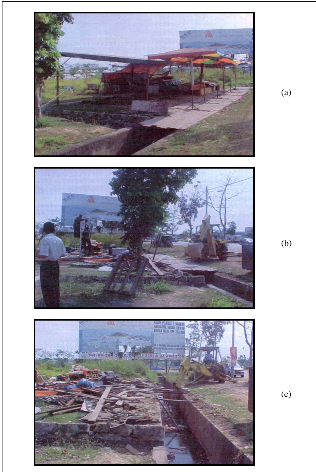
Figure E1 (a-c): Demolition of a seasonal fruit stall in progress. The temporary structure was built without valid permit and was considered trespassing on government land. The works were executed under the authority of Majlis Bandaraya Melaka Bersejarah.
