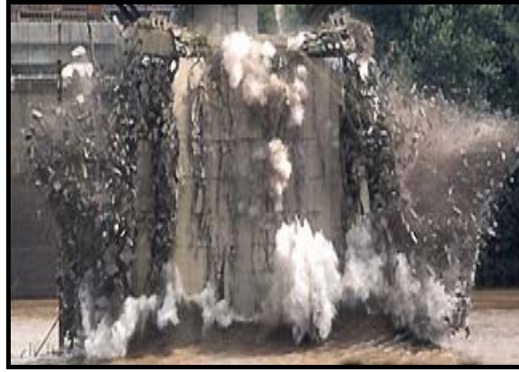
Figure 2.23: A shattering bridge pier (implosionworld.com, 2005).
