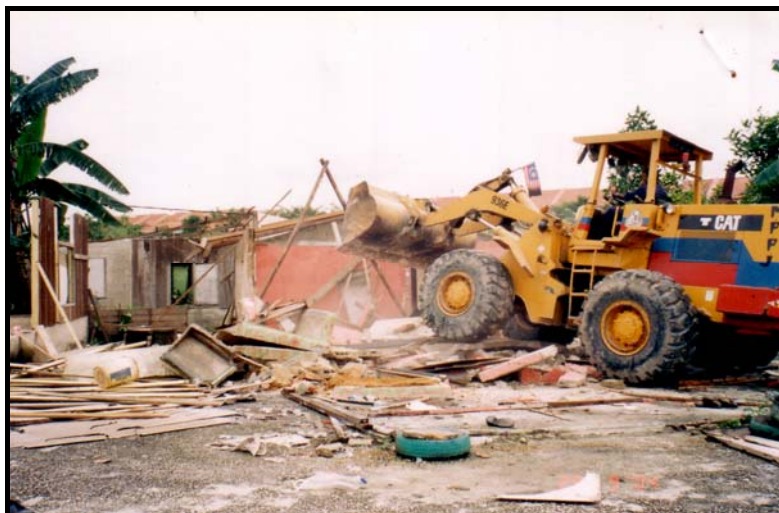
Figure E4: Demolition of squatter houses in progress. The works were executed under the authority of Majlis Perbandaran Petaling Jaya.
