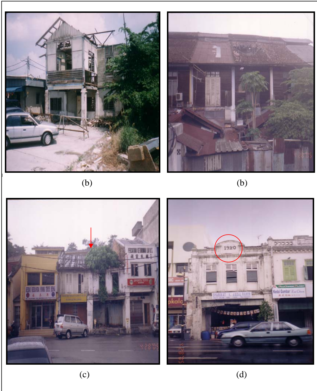
Figure D4 (a-c): These buildings have been abandoned and have deteriorated to such an extent that they are extremely dangerous. They not only become an eyesore but also provide excellent environment for drug addicts and pest breeding; (d) A clear indicator, (year 1920), reflecting the age of many existing buildings. All snapshots were taken in Seremban, Negeri Sembilan.
