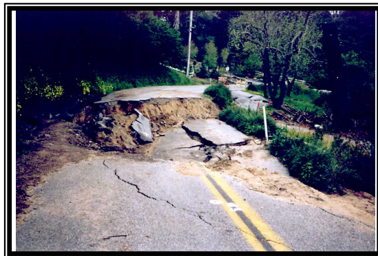
Figure 2.3: Road damage because of the landslide (Source: U. S. Geological Survey, 2001)
