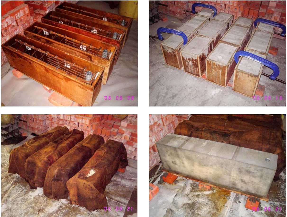
Figure 10 Preparation of precast concrete beams with sleeve: formwork preparation, concrete casting, curing and the completed specimen (from left, clockwise)
