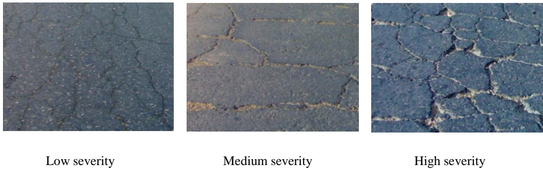
Figure 4.3 Severity levels of Alligator cracking
