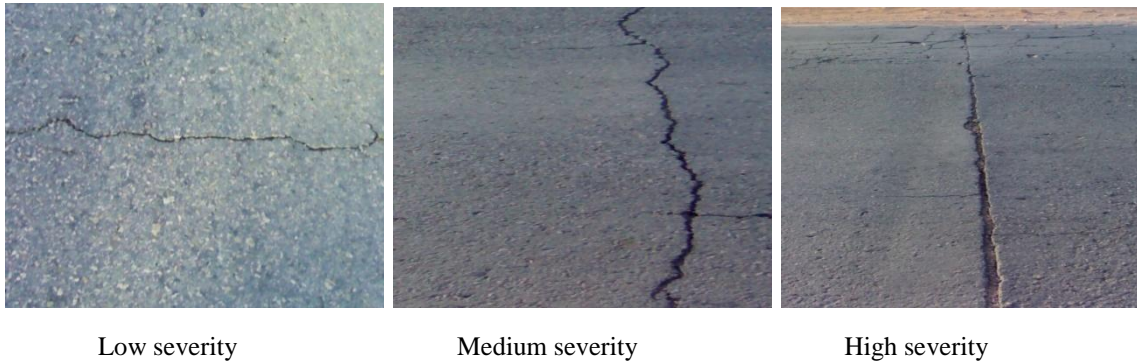
Figure 4.5 Severity levels of Transverse Cracks
