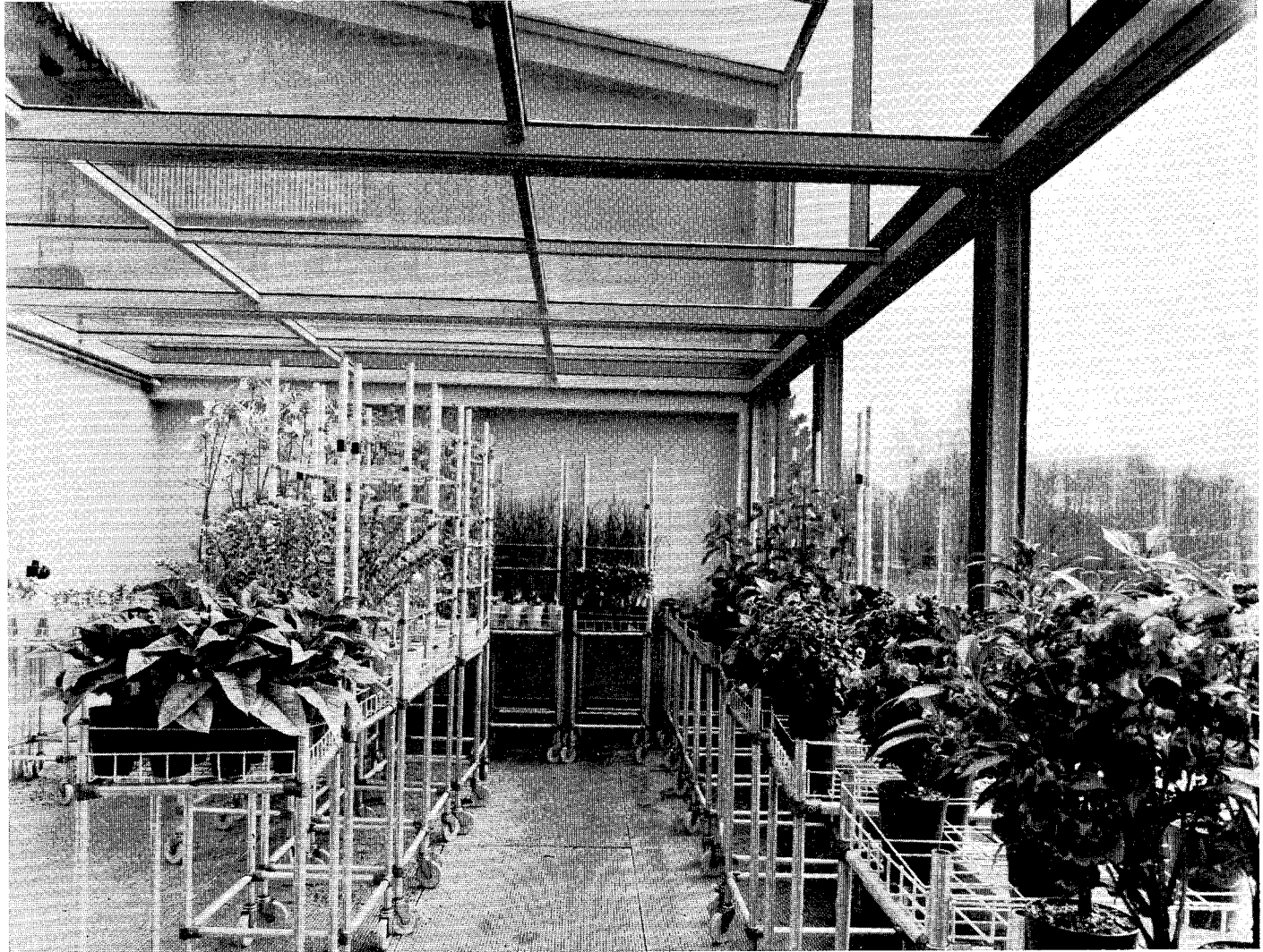
Fig. 2. Inside view of one air-conditioned greenhouse during use of daylight. The prepared air is blown through the perforated floor.
