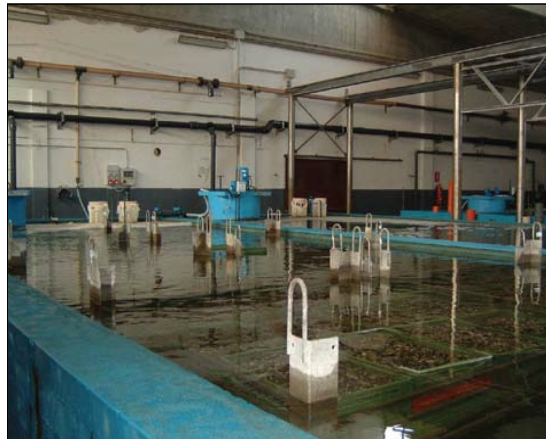
Fig. 1.3. Indoor mechanized Bivalve depuration plant.
