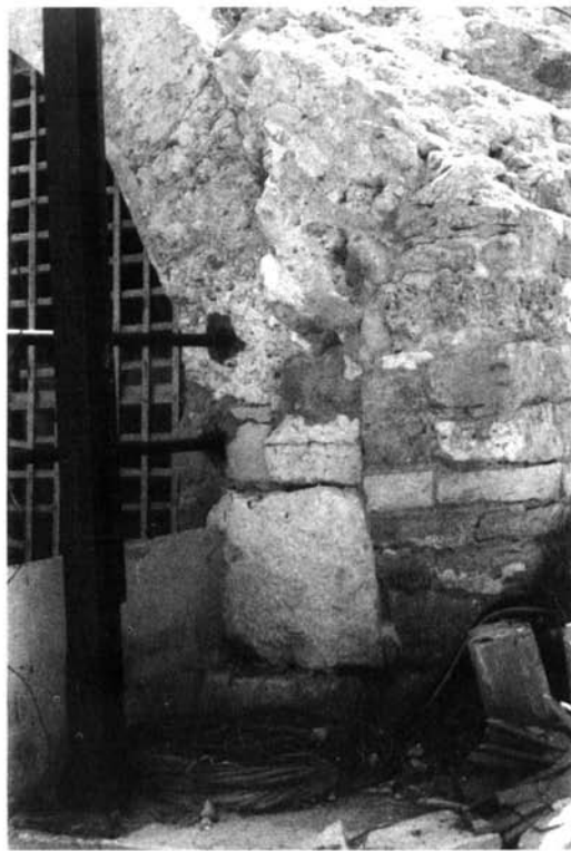
b - The south wall of the eastern aditus maximus . Only the lowest block (partially hidden by electrical cords) is in situ .
