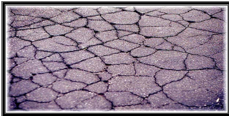
Figure (2-4): Flexible pavement distresses fatigue cracking (Bahia, 2006)
