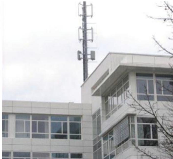
Figure 6.1.1-2: LTE antenna at Munich test site.
