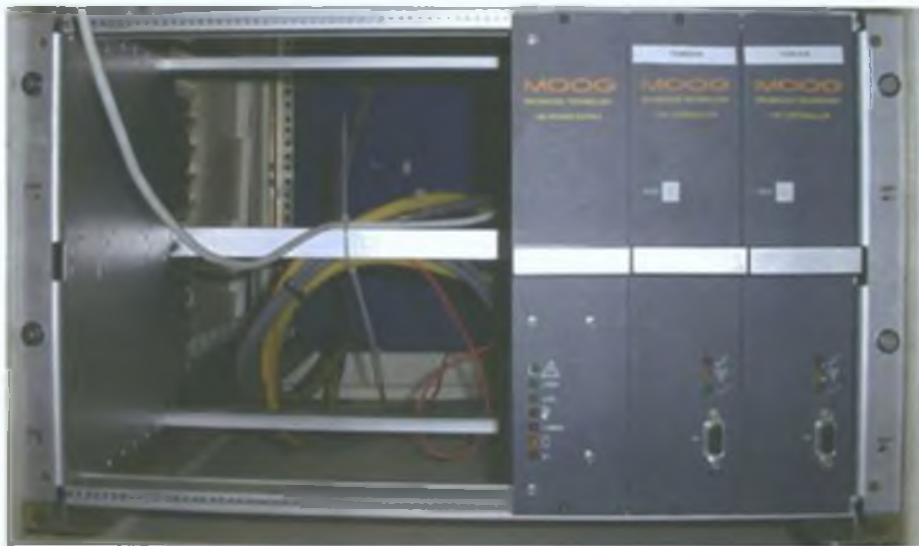
Figure 4.3 Controllers and Power supply rack
