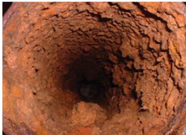
Figure 1.2, Corrosion on the internal walls of sour crude pipeline [4].
