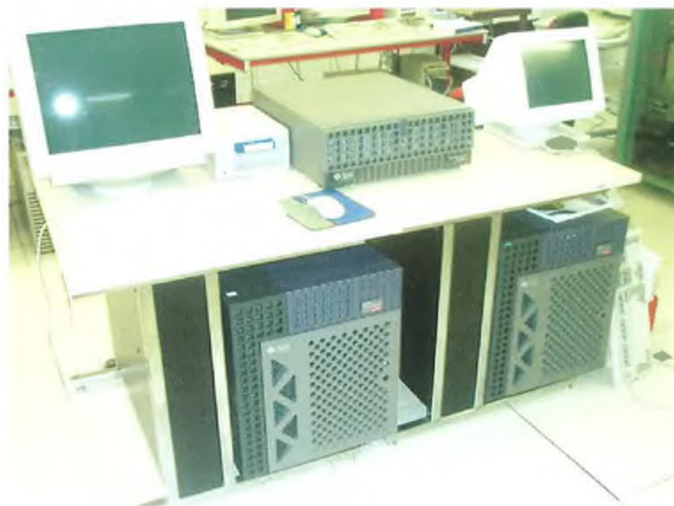
Figure 2.3 Depiction Of The Sun Microsystems Enterprise 450 Server Used To Host VPS Images.
