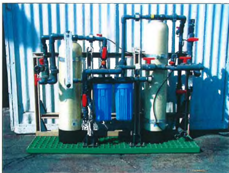
Figure 1. 5: Ion Exchange Equipment [24].
