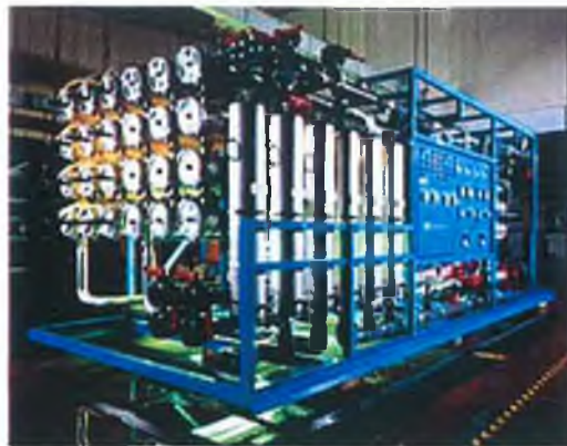
Figure 1. 7: Reverse Osmosis Equipment [27]
