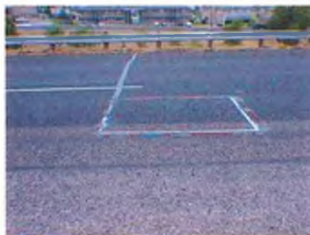
Figure 2.2: Induction loop embedded in a road
