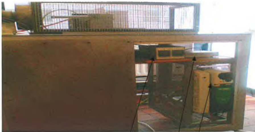
Figure E10 Temperature controller and motor controller with National Instrument data acquisition box
