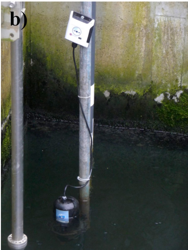
Figure 2: a) Effluent outflow tank, b) Phosphate analyser located below the water line and linked by cable to the communications module above.
