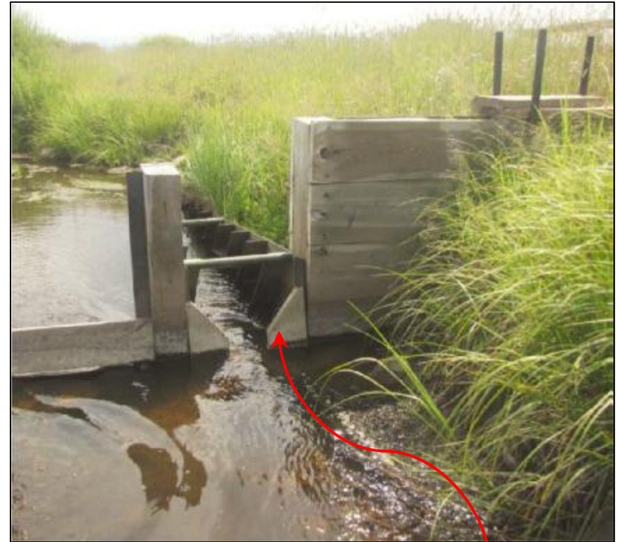
Flow Control Device in Field
