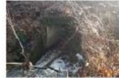
SR 99 concrete box culvert that blocked fish passage at West Fork Hyalison Creek near Tacoma.
