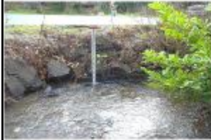
Before – undersized culvert
