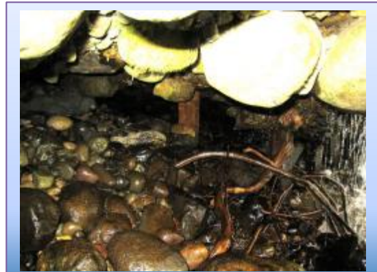
Undermining and exposed pile
