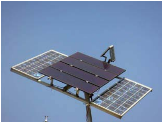
Fig.11: The combination of poly-crystalline PV modules (PhotoWatt PW 750) combined with amorphous PV modules (Free Energy Europe FEE-20-12) results in increased energy generation losses due to solar PV technology, size and brand mismatches.
