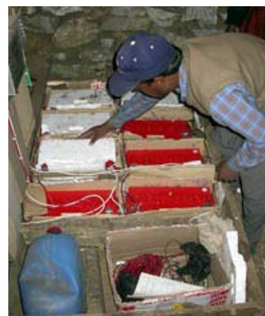
Fig.8: Installed Battery Bank
