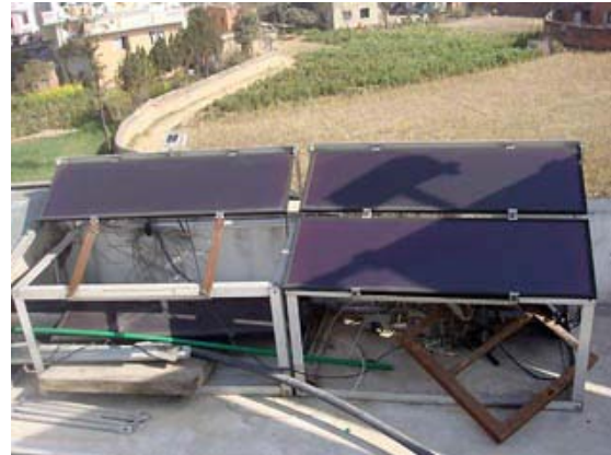
Fig.12: This amorphous PV Module (three Free Energy Europe FEE-20-12 modules) array's daily energy generation output is strongly affected by daily, long-term partial shading and insufficient free air flow around and through the array.
