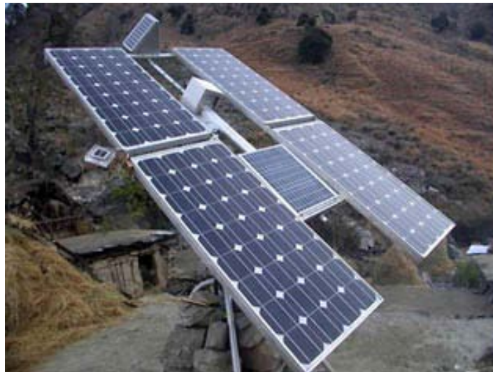
Fig. 3: One unit of the 2-Axis Solar Tracker in Humla with four BP 275F PV Modules
