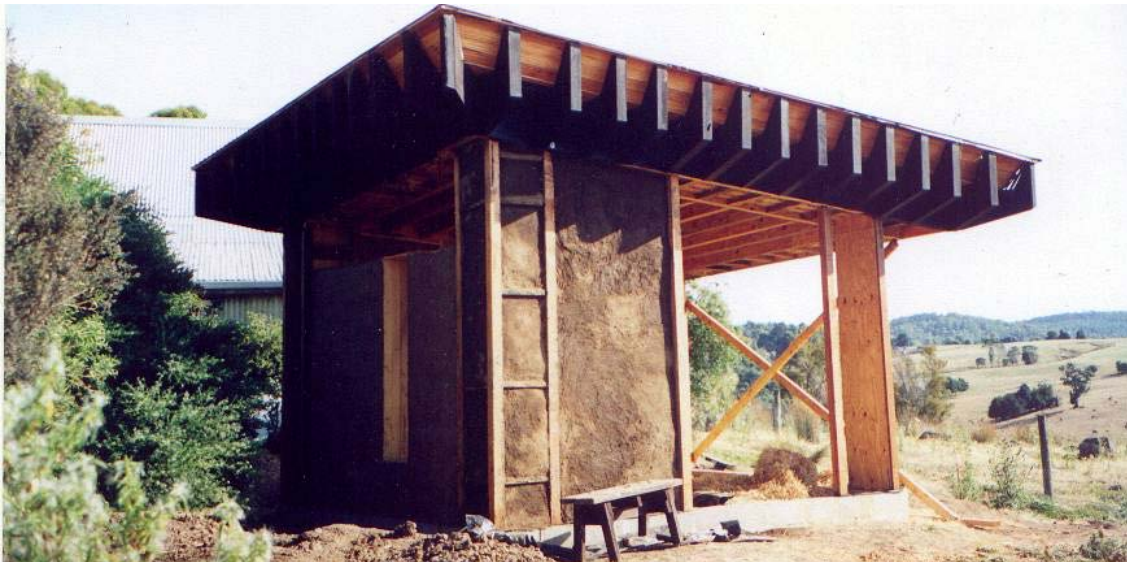
Image 11-12 After completion of straw bale infill and first layers of render (Richard Burnham, 2003)
