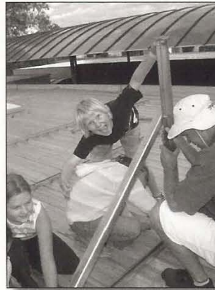
▲ Students installing the frames for the solar panels on the roof of the school.
