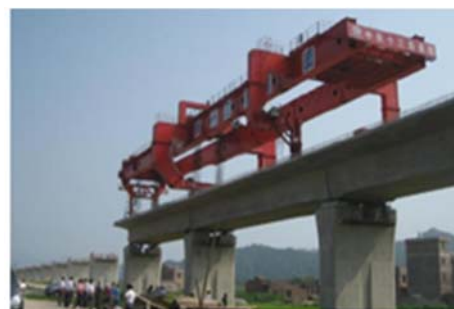
Beam Launching Equipment
