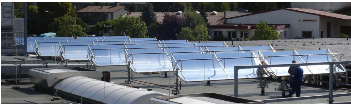
Fig. 1: Solar field with PTC1800 parabolic trough collectors
