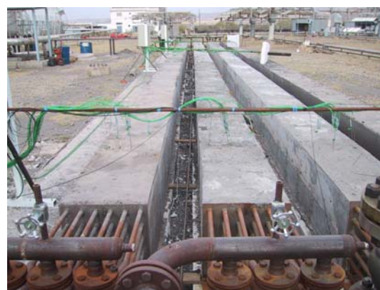
350 kWh concrete and cast ceramics test modules before mounting the thermal insulation
