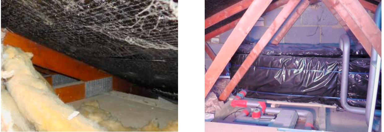
Figure 2: a) insulation missing above ceiling near eaves b) lack of insulation beneath cold water tank.
