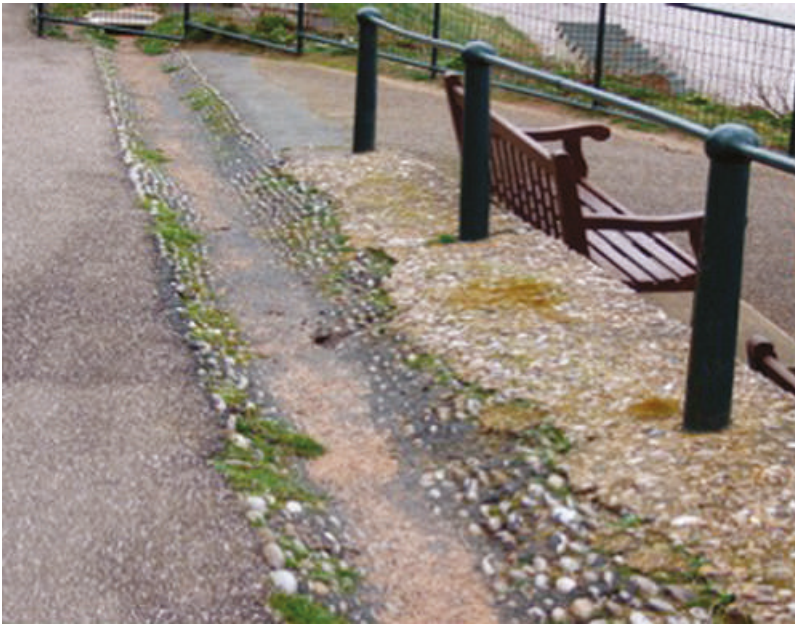
Figure 13.3a Budleigh Salterton seafront: drainage guttering (Source: author)
