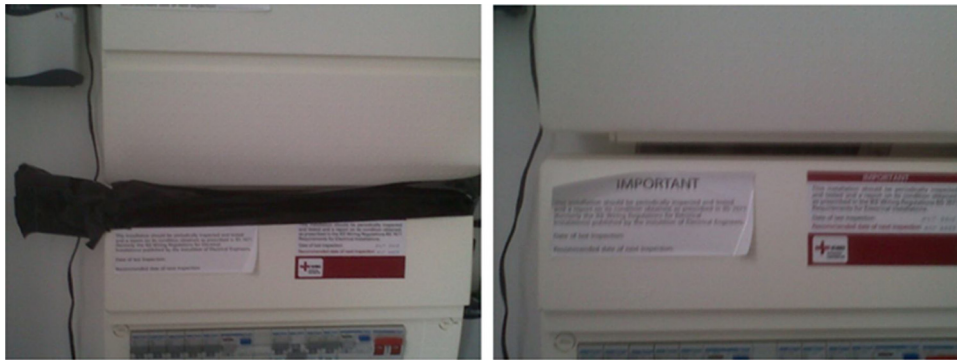
Fig. 1. Consumer unit as found by researchers immediately after an airtightness test (left) and the gap present when the adhesive tape was then removed (right).
