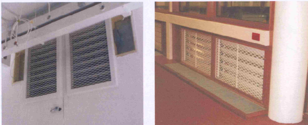
Figure 54: Components (a) high level vents to perimeter stack (b) low level inlets from central lightwell to occupied Spaces (Source: Cook et al.)
