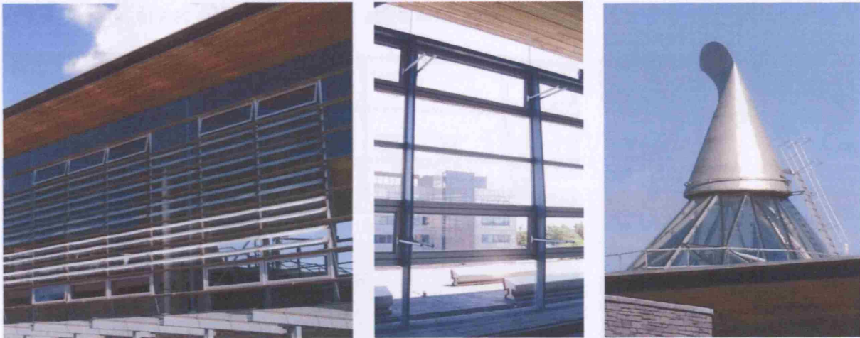
Figure 32: Ventilation components (a) west façade (b) view of actuators (c) wind cowl on the roof (Source: photo by author)
