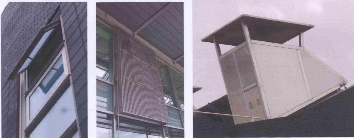
Figure 20: Ventilation components (a) Inlets on East and West façades (b) security grills (c) snout (Source: photo by author)
