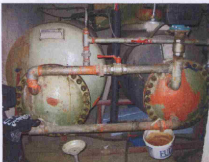
Figure 28: Hot water insulated storage tanks
