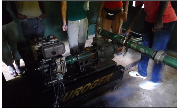
Figure 16. Motor-pump installed in Boma in 2009
