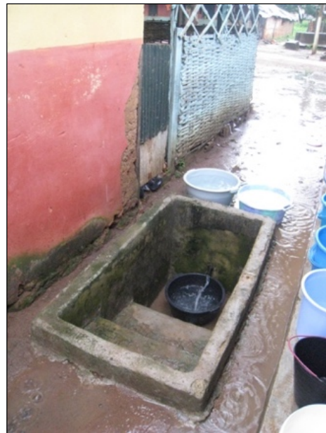
Figure 12. Home connection active in 2010 (before refurbishment works). The residents excavated a pit to overcome water pressure issues.
