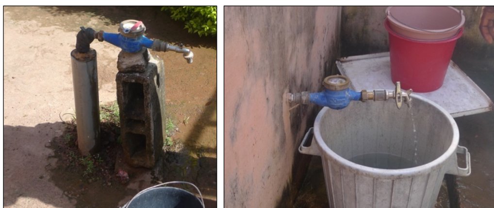
Figure 28. Home connections with meters and different devices to lock taps
