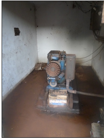
Figure 15. Pump installed in Bairro 4 in 2008
