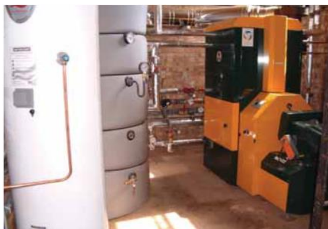
Figure A.10 Biomass boiler installation with wood pellet burner at Nayland Primary School, Suffolk (Source: Nayland Primary School, n.d.)
